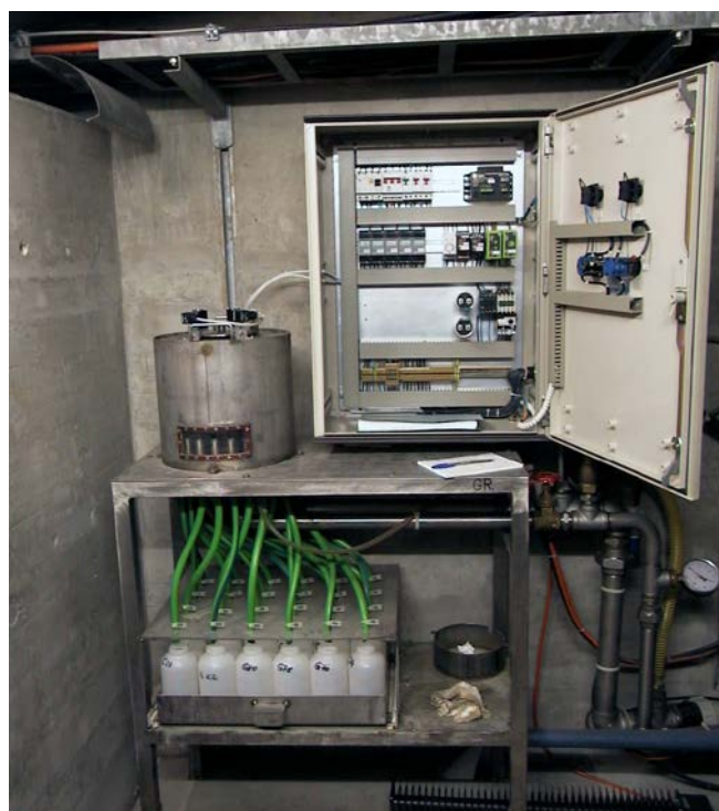
Figure 15 The automated sediment sampler (Verbund)
