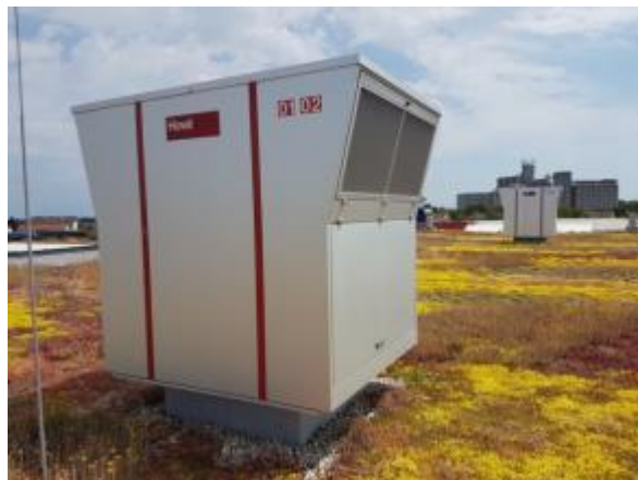
Figure 11: RoofVent RH units on the green roof (source: Pannonian wood competence centre gallery)
