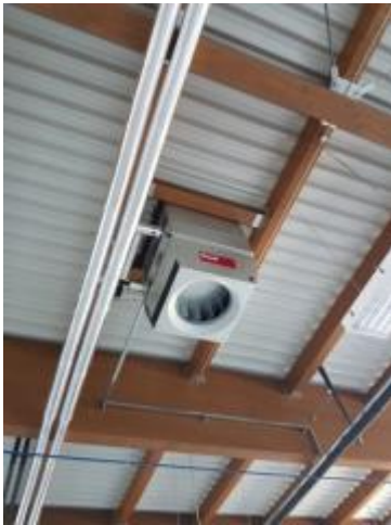
Figure 12: TopVent DHV unit inside the hall (source: Pannonian wood competence centre gallery)
