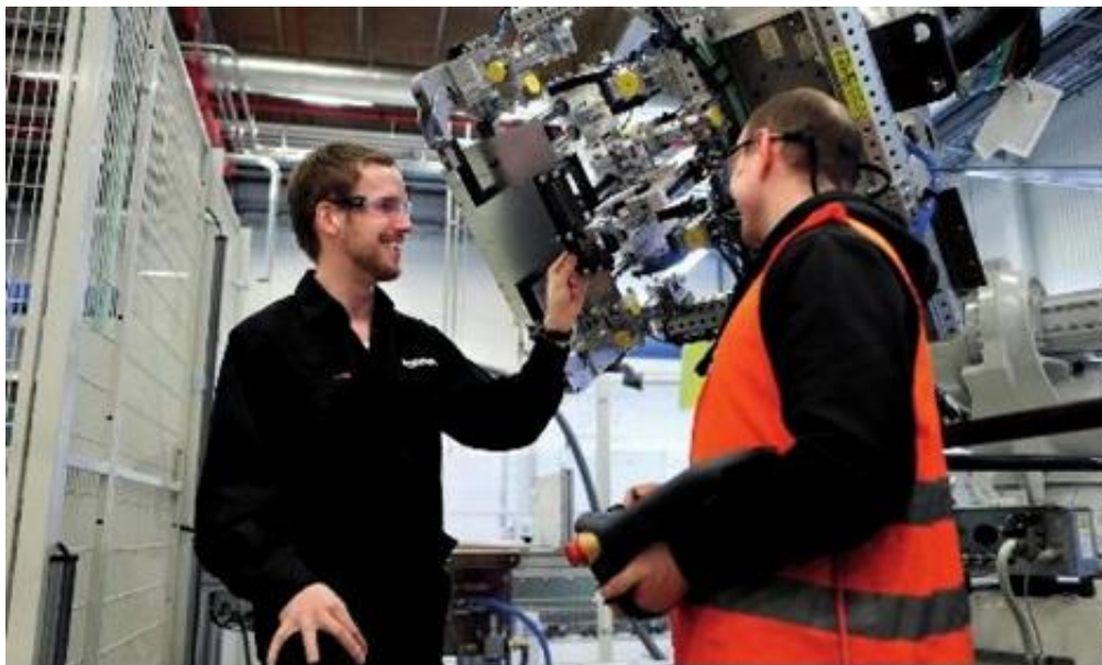
Figure: Robot commissioning
