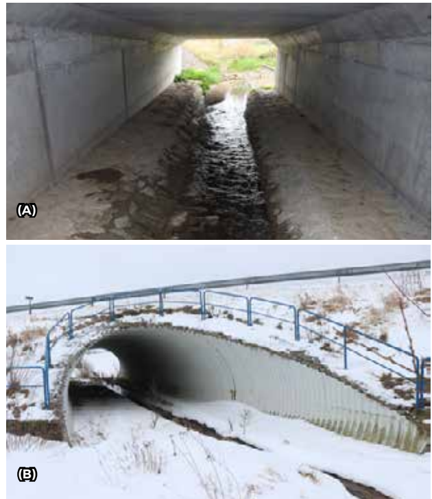
Fig. 10.42 Different types of bridges over small watercourses are very well usable as fauna passages for small animals. Dry banks at least 0.5 m wide allow the movement of a broad spectrum of species up to the size of badger. The banks should be made from stone pavement and concrete should be avoided, because it does not allow migration of amphibians (risk of drying out). © Václav Hlaváč
