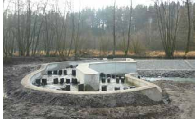
Fig. 10.49 A fish crossing in the form of a bypass - in order to overcome a weir 1.3 m high, it was necessary to create a fish crossing with a total length of 40 m. The Czech Republic. © Bohumila Jermlová
