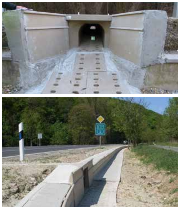
Fig. 10.48 An amphibian tunnel is a good solution for overcoming narrow roads of lower category. Barriers guiding animals to the passage are a necessary condition for proper functionality. © András Weipert
