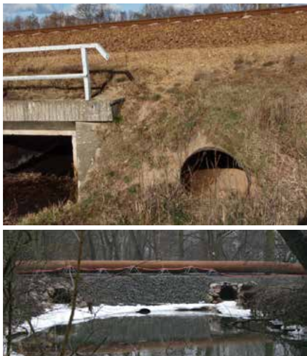
Fig. 10.47 Otter tunnels are a suitable solution in places where a bridge is impassable for otters or where transport infrastructure is led on top of a pond or reservoir dam. © Lukáš Poledník
