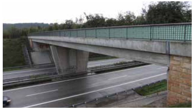
Fig. 10.30 A bridge for a forest path over a motorway was in this case widened by 2 m on each side and the new strips were planted with bushes. Disturbances are eliminated by protection walls (full railing). Such a multi-purpose overpass can be used by smaller mammal species (up to the size of fox or badger), but also by small birds, bats, tree top species, etc. Germany. © Václav Hlaváč
