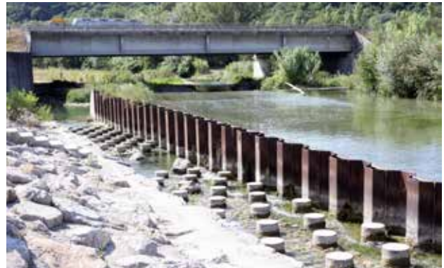
Fig. 10.50 A fish crossing near Lyon, France, where a vertical step on a watercourse was created as a result of a road construction. The fish crossing is placed directly in the watercourse and is used by the entire fish spectrum inhabiting the stream. It is also used by otters. © Václav Hlaváč
