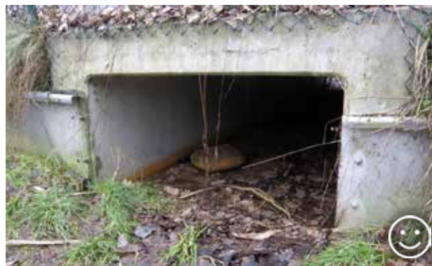
Fig. 10.43 Rectangular culvert is a good solution for amphibians, reptiles and mammals up to the size of fox or badger. © Lukáš Poledník
