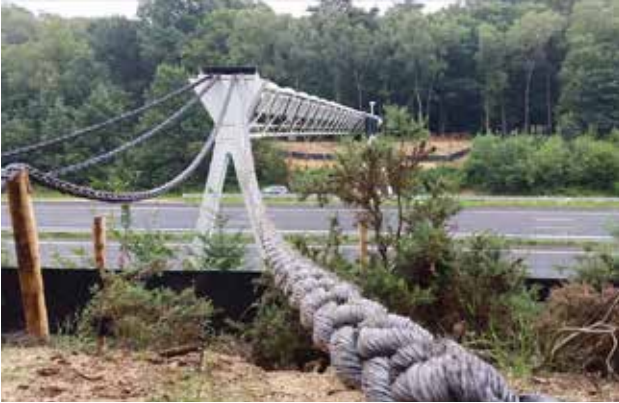
Fig. 10.16 Example of a special passage for mammals living on trees: a gantry over the A12 motorway (Utrecht - Arnhem, near Wofheze, the Netherlands) adapted for use by the pine marten. The gantry contains a "walk-path" and thick ropes connect it at both ends to the edge of the nearby forest. Use by the species has already been proven by a phototrap. © Jan Willem Burgmans, Heijmans Infra
