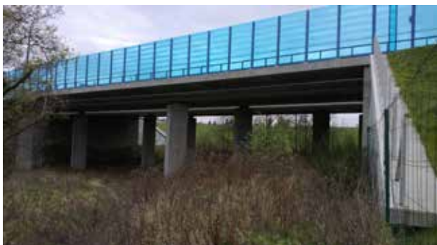
Fig. 10.38 Natural surfaces significantly improve the functionality of a wildlife underpass. A protection wall contributes to better utilization by fauna as well, thanks to disturbance elimination. A transparent wall has to be secured against bird injuries. The Czech Republic.
