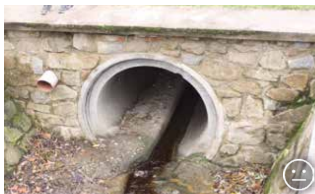
Fig. 10.44 Usability of culverts for animals can be increased by creating a dry concrete bank which allows for the movement of terrestrial animals. © Václav Hlaváč
