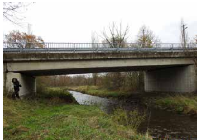
Fig. 9.9 Properly designed bridge over a stream with dry banks that allows for movement of most animal groups. © Lukáš Poledník
