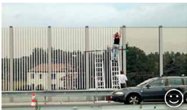
Fig. 10.60 The process of installation of glued stripes to a noise protection wall on D47 motorway in the Czech Republic. In 2008, almost 200 dead birds were found along just 1 km long stretch of this motorway between Bohumín and Ostrava within 6 months. This mortality rate dropped practically to zero after equipping the wall with the stripes. © Jan Mayer
