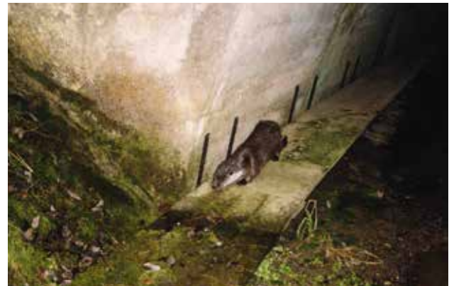
Fig. 10.13 In the case of bridges without dry banks it is possible to create additional "animal ledges." The natural continuity of the "path" to the stream banks must be maintained. © Václav Hlaváč
