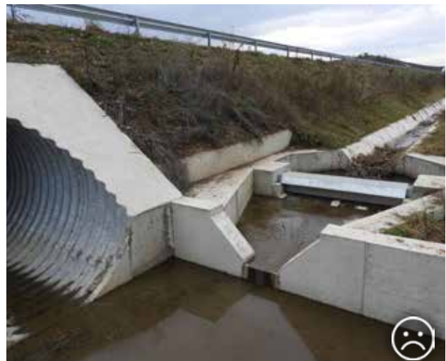
Fig. 9.18 Culverts of larger diameter should always be adapted for passage of fauna under a motorway as well. The outflow is in this case technically arranged in a way that completely eliminates the possibility to use the culvert as fauna passage. In addition, it can create a deadly trap for small animals (amphibians, small mammals) trying to pass through. © Václav Hlaváč
