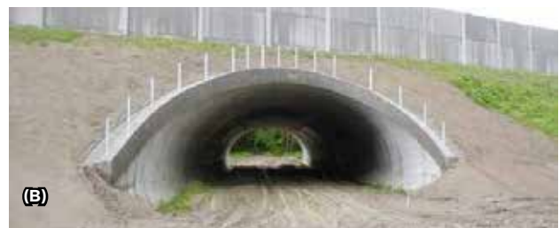
Fig. 10.37 Behaviour of animals near underpasses makes it evident that they register the noise caused by the passing vehicles (bearings of the bridge plate) - (A). Therefore, while constructing new bridges, it is always necessary to choose a solution that minimizes noise under the bridge. Noise under a bridge is best eliminated when there is a layer of soil between the bridge construction and the road/railway (B). However, this solution always brings under comparable conditions a reduction of the bridge dimensions as well. © (a) by Friends of the Earth Czech Republic, photo (b) by Nature Conservation Agency of the Czech Republic
