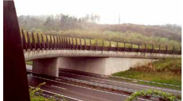
Fig. 10.24 Funnel shaped green bridge may be 40 m wide at the entrances, but only 10 m wide in the middle. This solution means financial savings without a significant influence on functionality. The picture shows the same overpass as in Fig. 10.23 in Luxembourg. © Václav Hlaváč.
