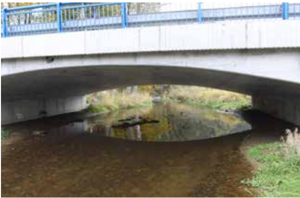
Fig. 10.8 Birds such as the common kingfisher, the white-throated dipper, or the grey wagtail are able to fly under a bridge with the openness index of at least 1-2. Height is also important; it should be minimally 2 m. In case of bridges with smaller dimensions birds typically fly over them and often become traffic victims. © Václav Hlaváč
