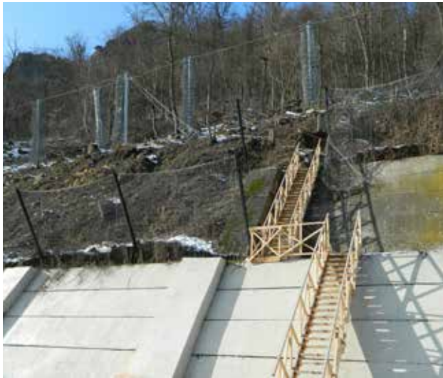
Fig. 9.13 Steep slope secured by a catch fence or wire mesh against falling stones. These measures are sometimes necessary to stabilize slopes, but at the same time they represent a reinforcement of the barrier effect and the destruction of road verges as natural habitats. If possible, a more gentle solution should be preferred. R2, Zvolen, Slovakia. © Miroslav Jarný
