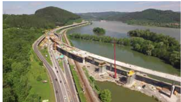
Fig. 8.10 Construction of a motorway parallel with road of lower category, railway or a river channel creates multiple barrier effect. © NDS Archive
