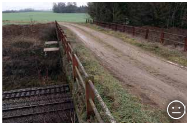
Fig. 10.2 A multi-purpose overpass over a double-track railway Prague - Brno (Czech Republic) is 7 m wide and 35 m long. Grassy stripes on the sides are used by a broad spectrum of invertebrates. Thanks to a clay surface the overpass is regularly used by the roe deer, the hare, the fox and many other species of small vertebrates, including the sand lizard. Similar bridges over motorways are used only exceptionally, because the disturbance coming from traffic is much more intense there compared to a railway. © Václav Hlaváč
