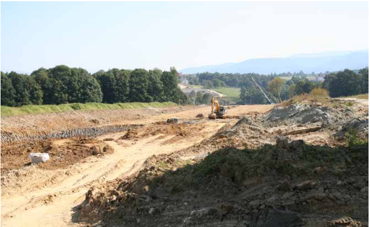
Fig. 4.1 Construction of roads in mountain environment often brings destruction of valuable habitats. Road S52 between Skoczów and Bielsko-Biała, Poland. © Ivo Dostál
