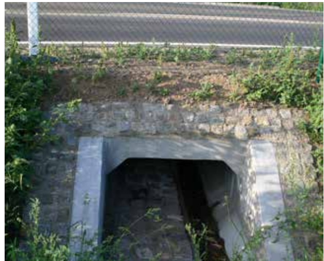
Fig. 9.5 Rectangular culverts suitable for passage of mammals up to the size of fox and badger are relatively easy to build on infrastructures in flat landscapes. © Lukáš Poledník
