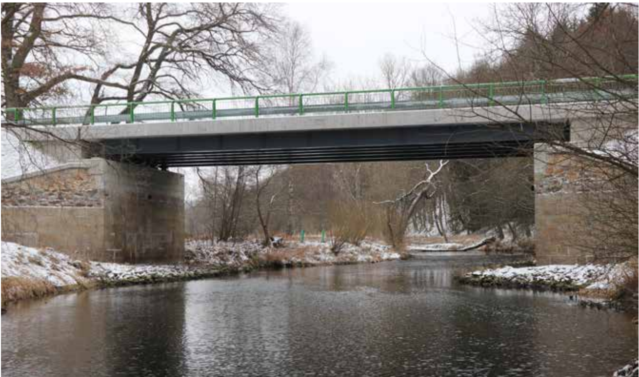
Fig. 10.1 Bridges over watercourses can easily be adjusted in a way that allows animals to use them to safely overcome a road. It is necessary to keep natural banks that fluently continue in the surrounding terrain. © Václav Hlaváč
