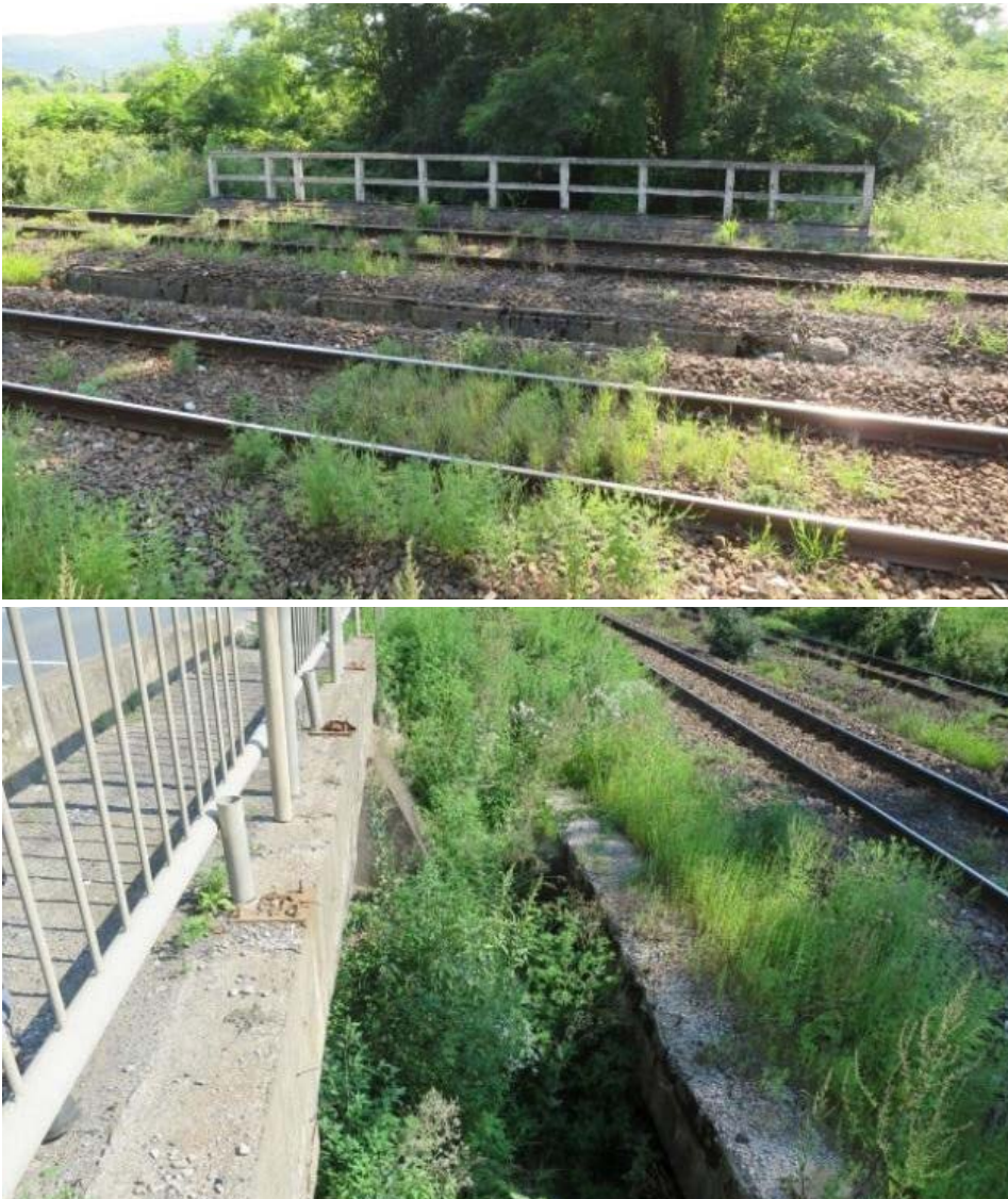
Fig 12. Example of blocked small bridge/culvert on the existing railway - Km 566+100
