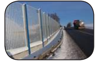
NOISE PROTECTION WALL SECURED FROM BIRD COLLISIONS
