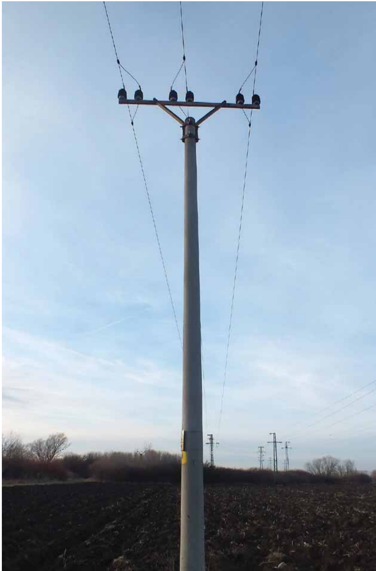
Fig. 6: Medium risk: Electric pole with a pair of support insulators in vertical position on console. © Raptor Protection of Slovakia
