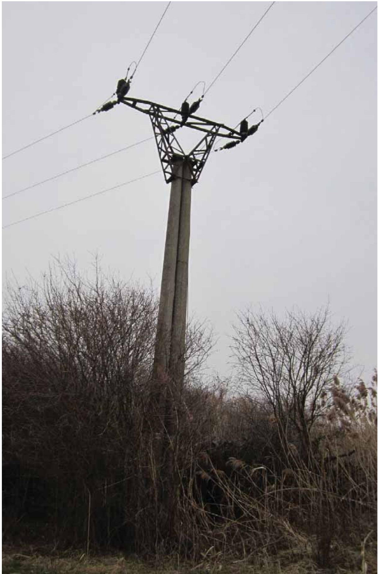
Fig. 4: High risk: Electric pole with three exposed jumper wires above the console. © Raptor Protection of Slovakia
