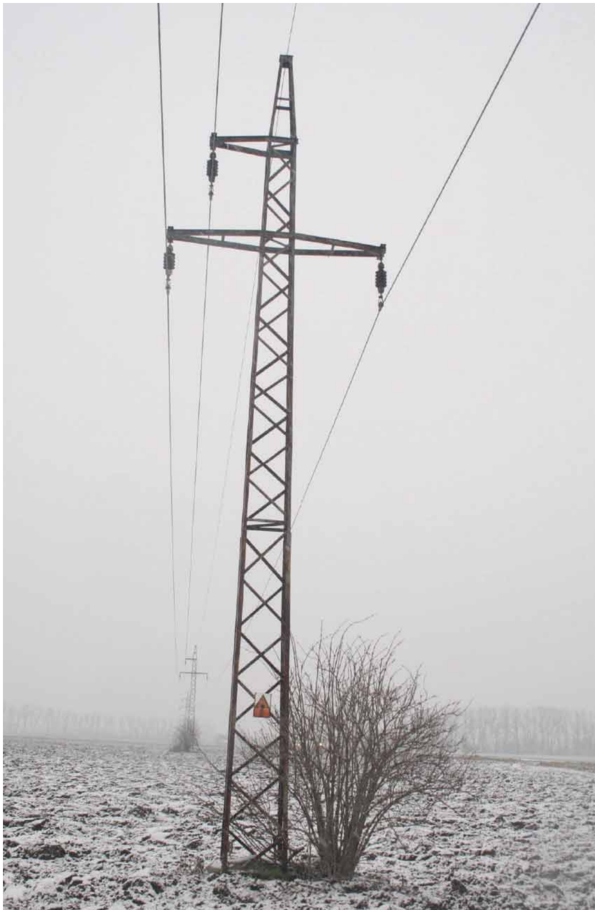
Fig. 12: Low risk: Electric pole with hanging insulators. © Raptor Protection of Slovakia
