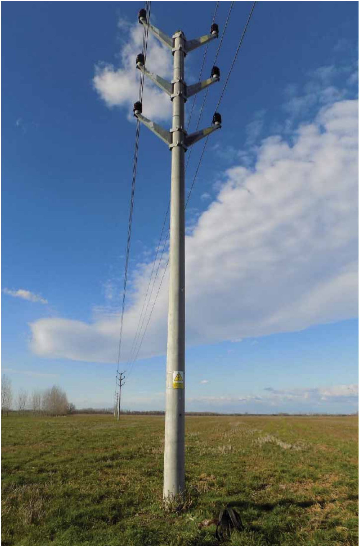
Fig. 13: Low risk: Double circuit electric pole with 45° angle of the arms. © Raptor Protection of Slovakia
