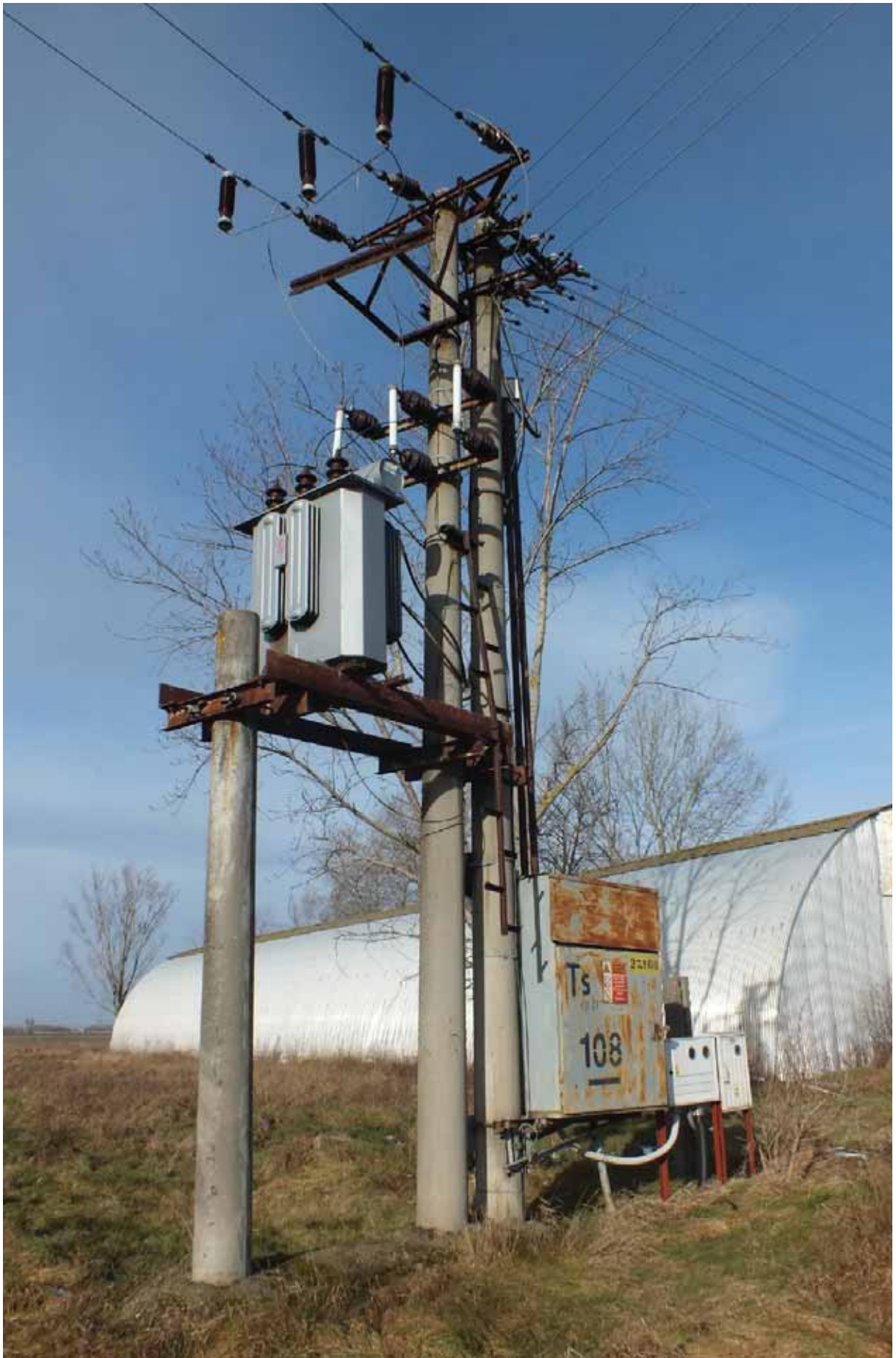
Fig. 7: Medium risk: Electric pole transformer with a combination of exposed jumper wires locations. © Raptor Protection of Slovakia
