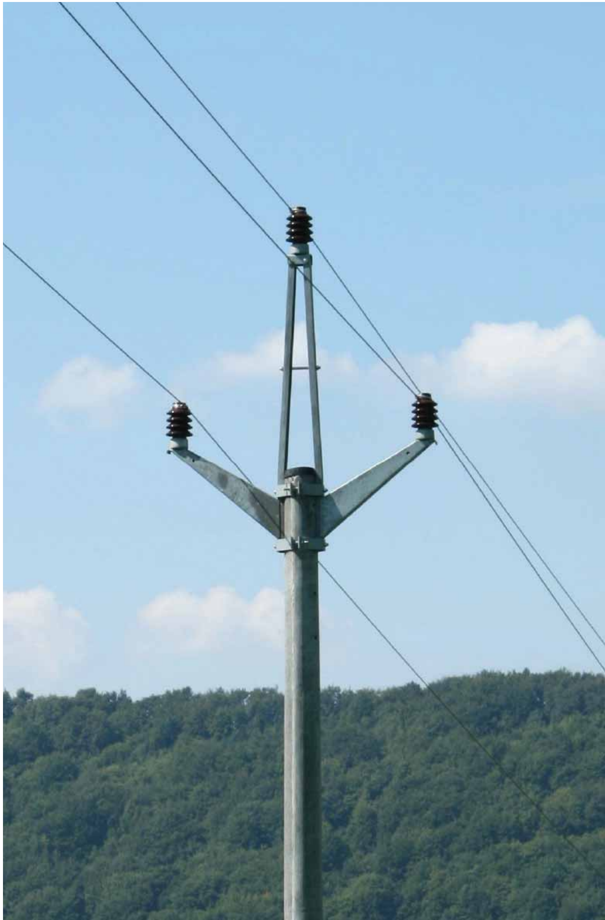
Fig. 10: Low risk: Electric pole with 45° angle of the arms. © Raptor Protection of Slovakia
