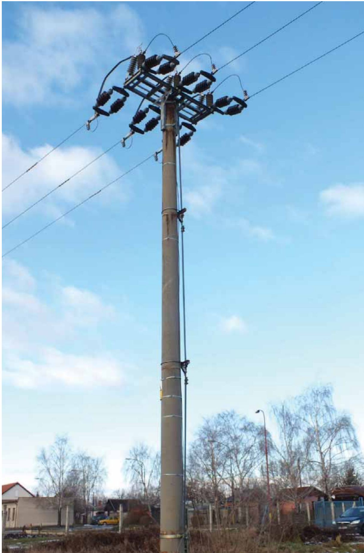
Fig. 8: Medium risk: Power line switch disconnecter. © Raptor Protection of Slovakia
