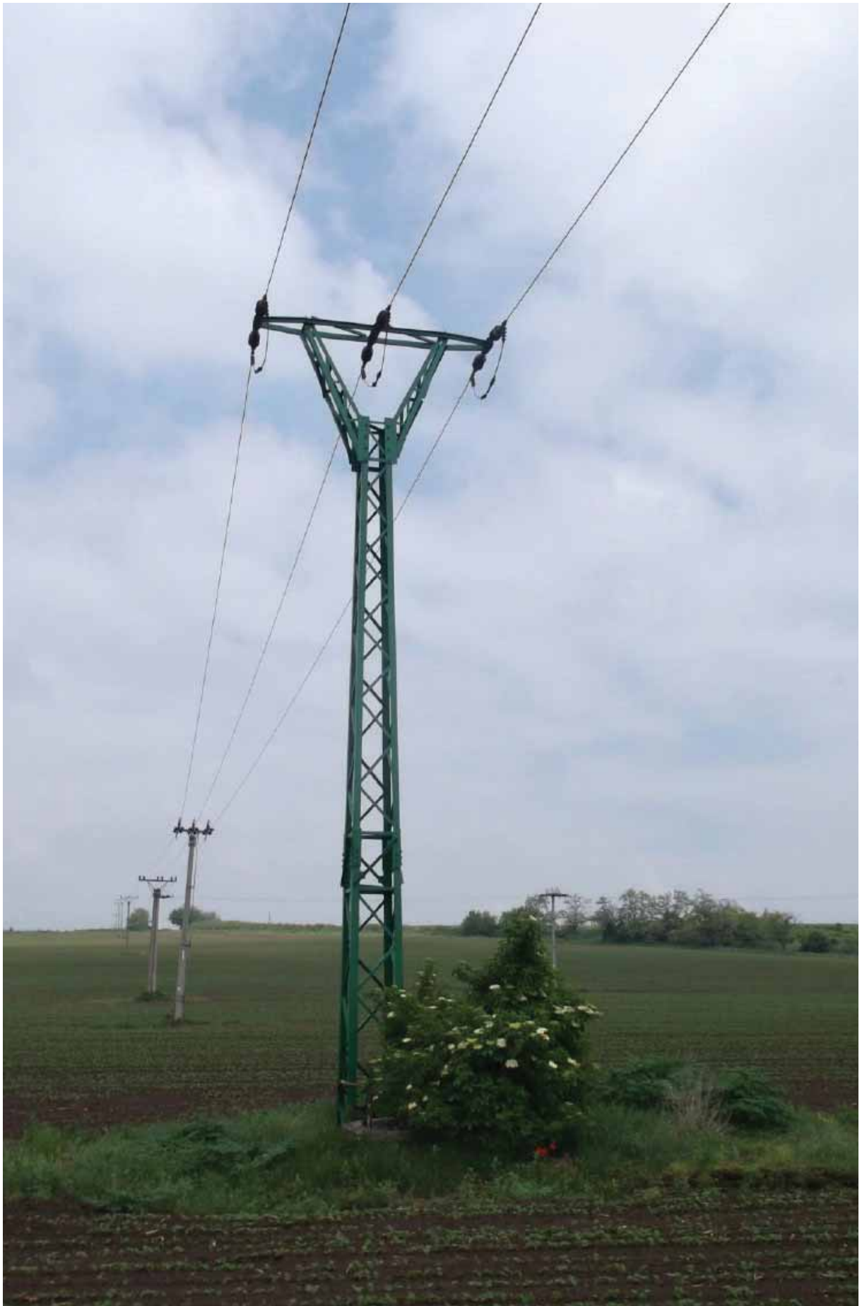
Fig. 9: Medium risk: Electric pole with hanging exposed jumper wires below the console. © Raptor Protection of Slovakia
