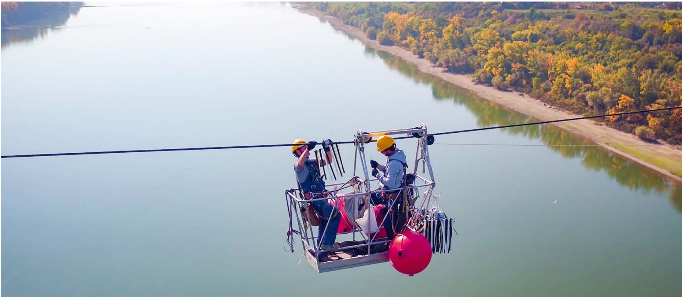
Close cooperation with the electricity providers: Marking of a high-risk power line crossing the Danube in Hungary.
