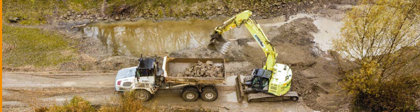
Tangible pilot actions improved river dynamics: side arm restoration through the removal of artificial groynes in Austria.
