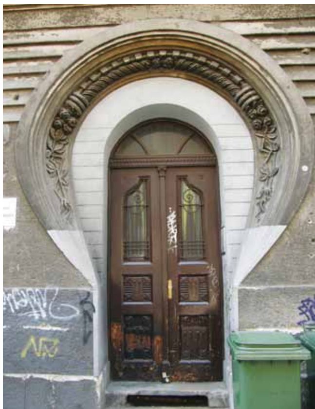
5. 20 Đorđićeva Street: Stucco decoration around the main entrance, before the restoration
