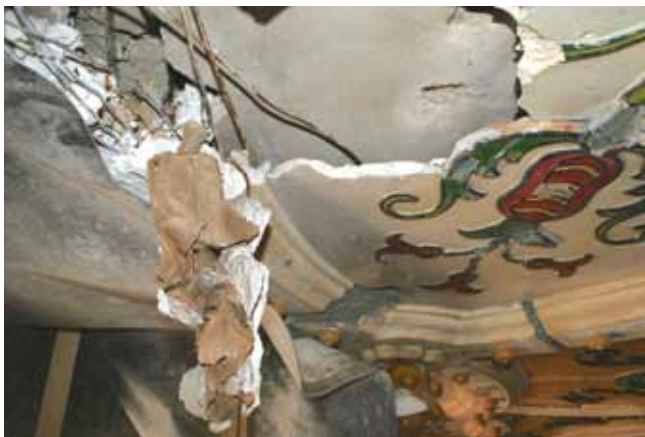
10. After the cleaning and the removal of the ceiling ceramics in bad condition, the problems turned out to be critical
