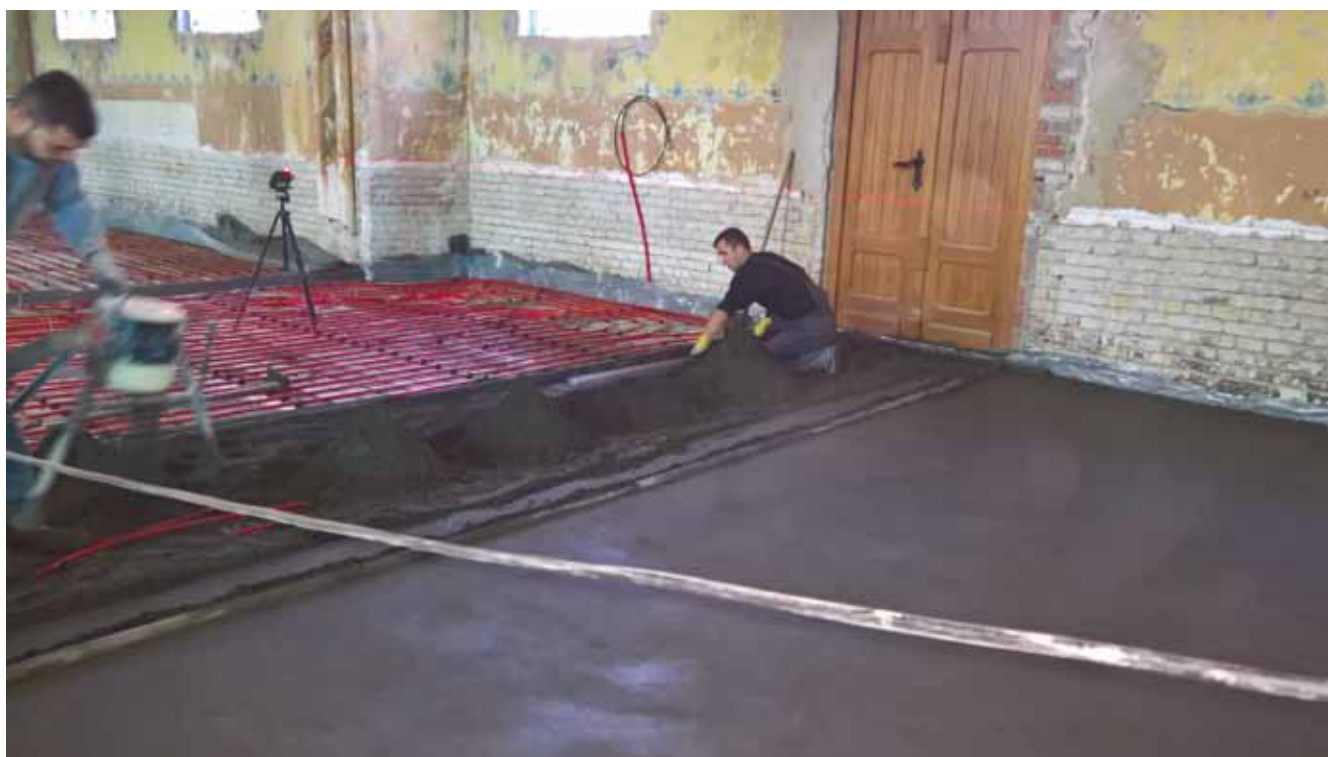
5. Under-floor heating through a system of pipes
