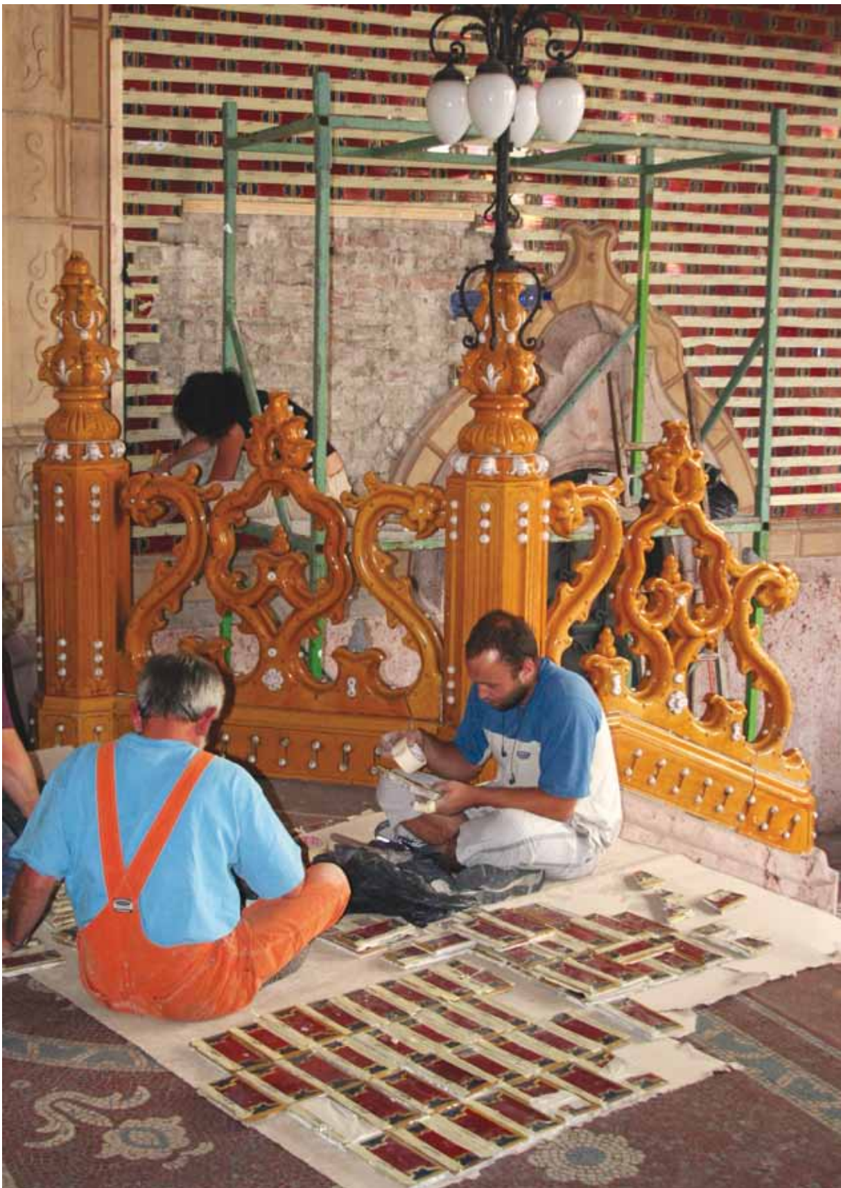
7. All the removed tiles were properly cleaned, and damaged tiles were taken to our workshop for further restoration processes
