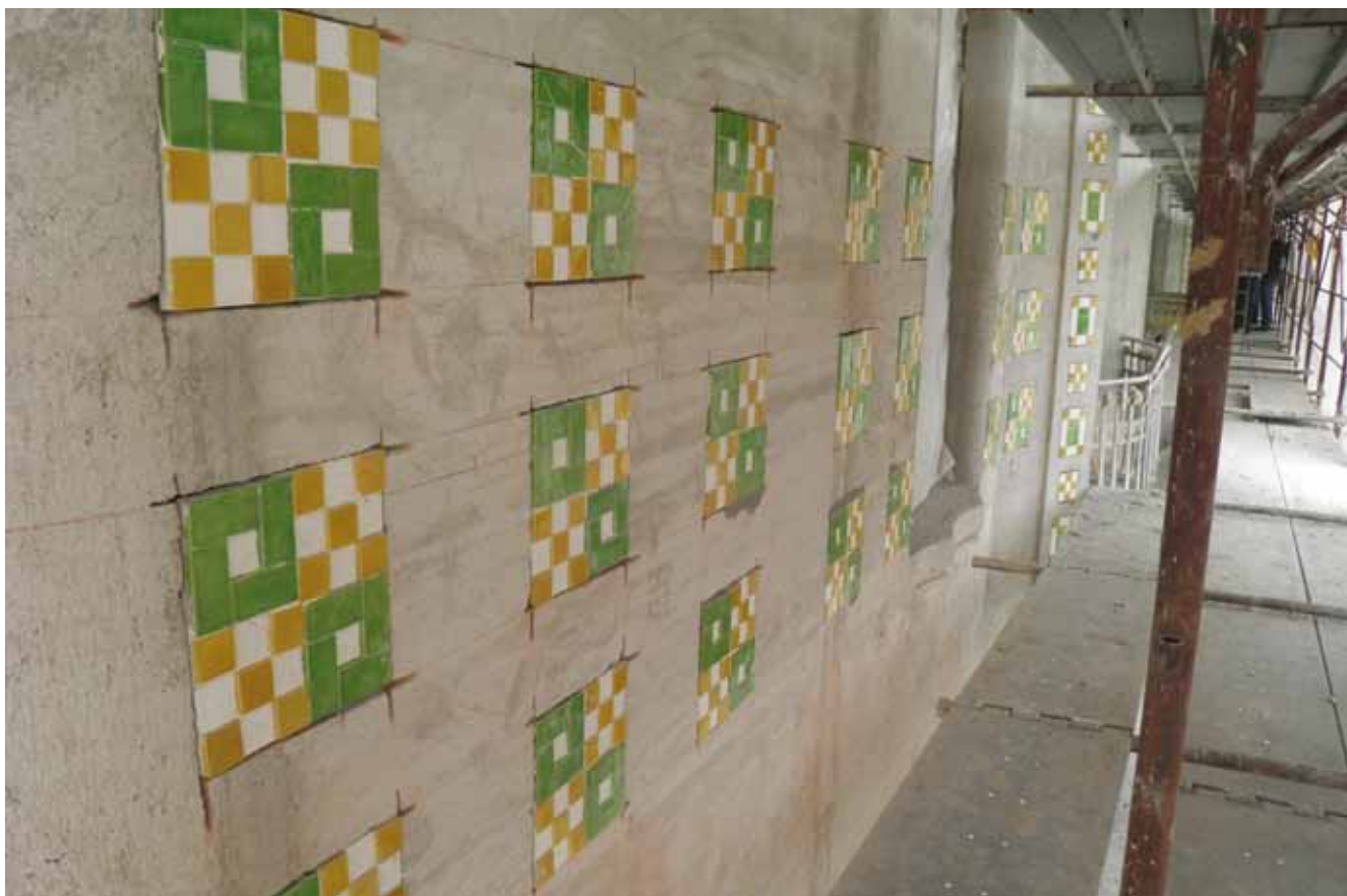
12. Adolf Moskovits Palace, the new plastering is made even with the slabs bearing the ornaments
