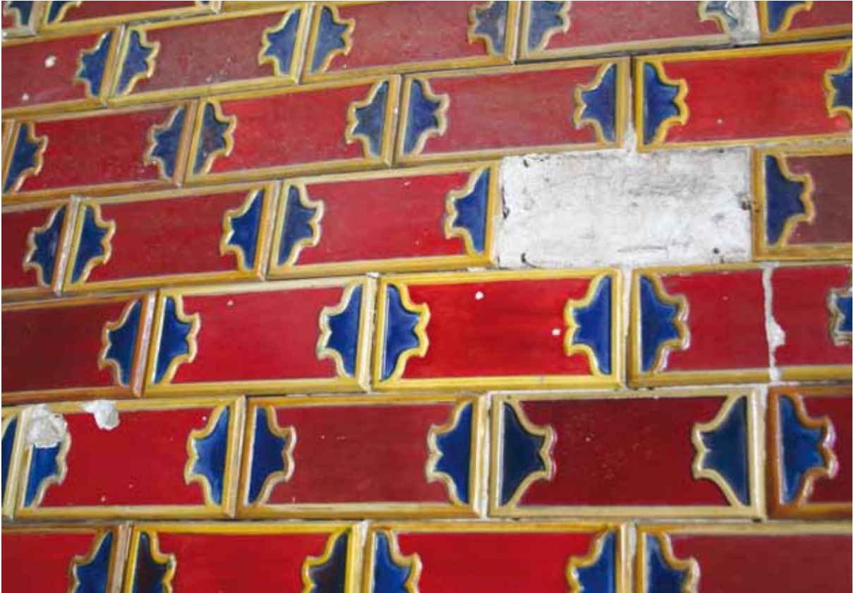
5. Decorative elements with ruby-colored luster glaze. The types of damage: gunshots, mechanical damage, damage due to leaks and fractures due to tension
