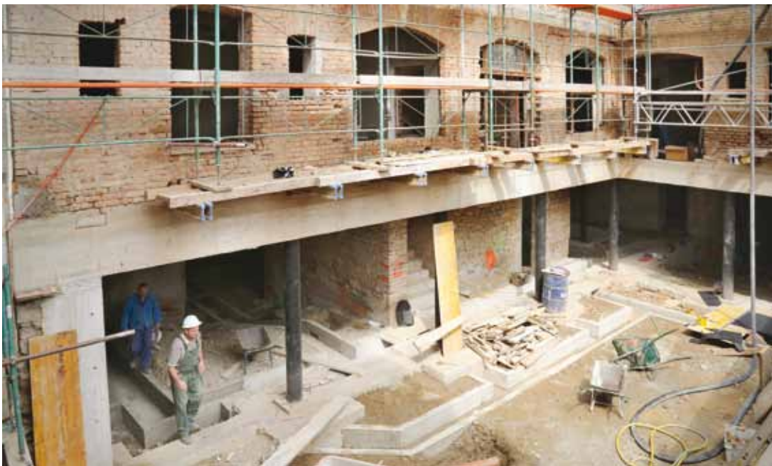
8. The entire basement level has been deepened and extended in order to incorporate the courtyard
