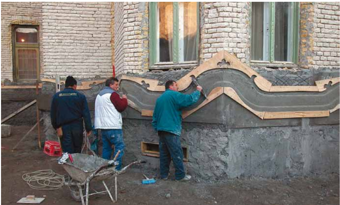
10. Restoration work on the courtyard façade using templates to make the undulating plaster forms
