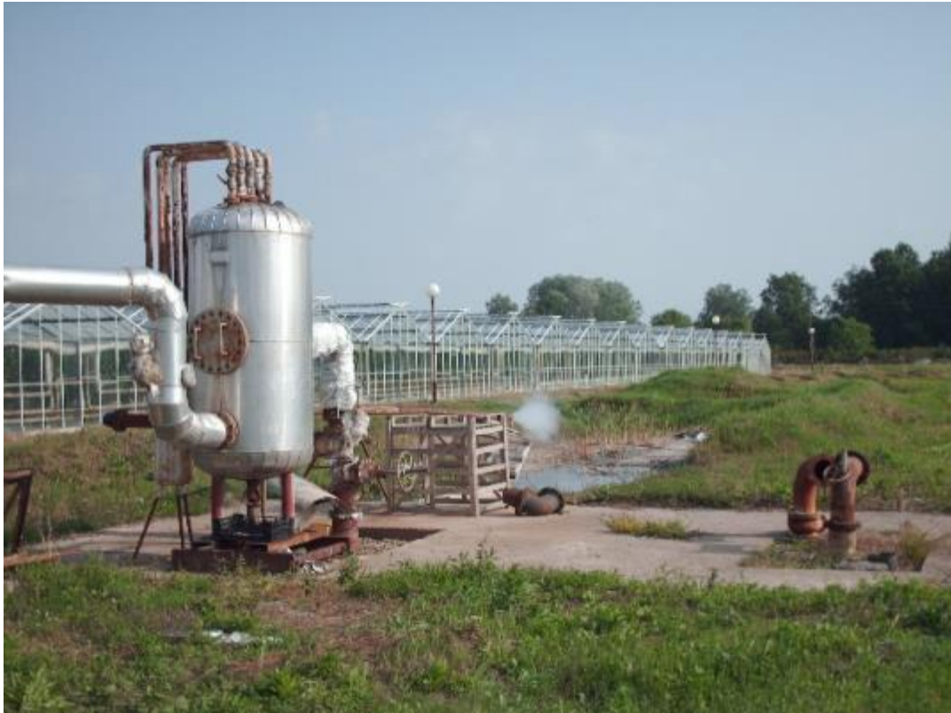
Figure 20: Well Do-3/B in operation in 2007 (Photo: Natalija Samardžić)
