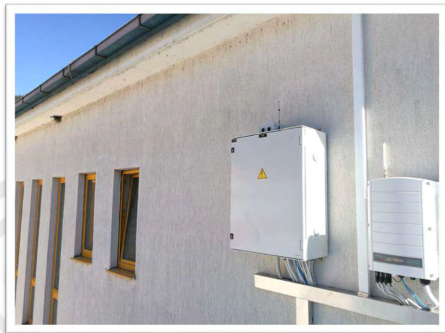
Electrical installations cabinet and inverter box
