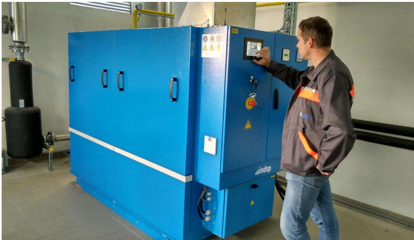
CHP unit in boiler room
