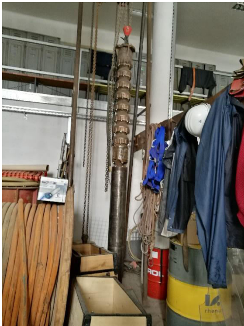
Figure 3.3.2: Spare water pump.
