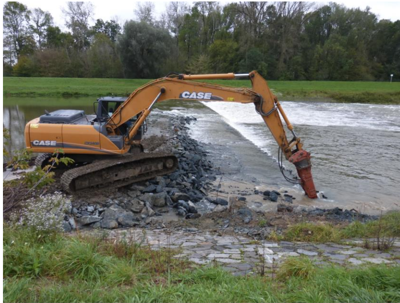
Figure 10: Removal of the substructure of the original tube weir on the river Morava
