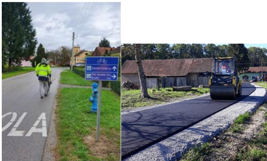
17-18. Figures: Just installed signpost in stage S8 (left); new asphalted road in Brodić (right)
