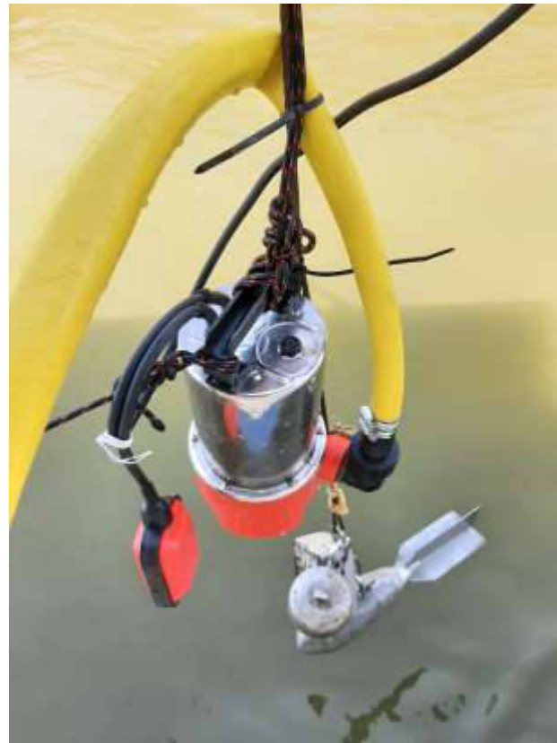
Submersible pump (close view)
