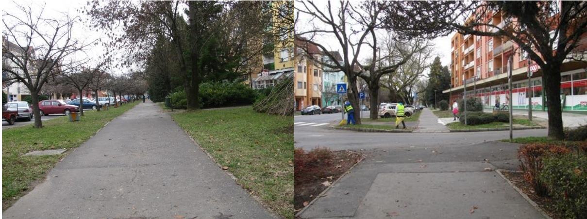
35-36. Figures: trace of the new bicycle path inside Nagyatád (currently under construction)
