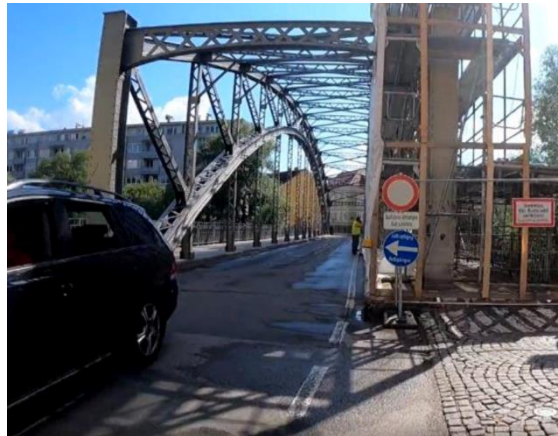
Problematic traffic signs at construction site, with not safe detour route at EuroVelo 14 in Austria
