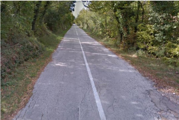
Potholes and damage due to tree roots at EuroVelo 8 in Croatia
