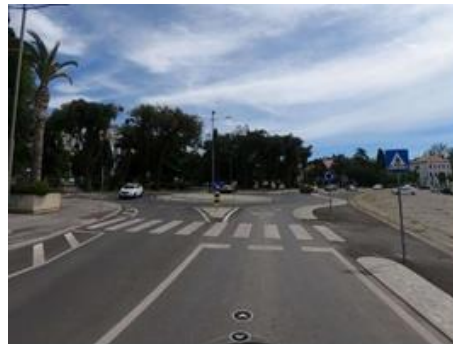
This roundabout in Pula, Croatia, has recently been built, and even though cyclists can be frequently seen along this road section, no infrastructure has been dedicated to them (EuroVelo 8).
