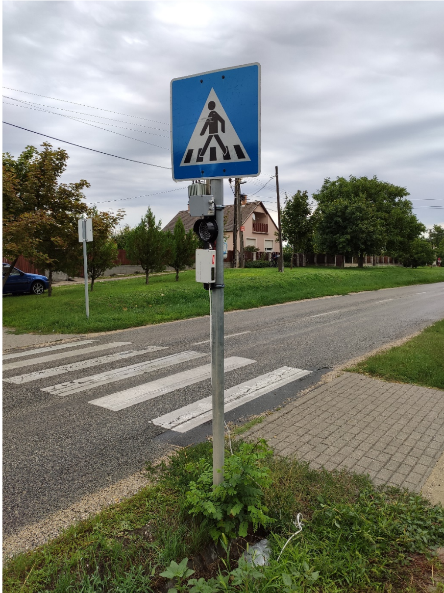
Figure 2: The yellow blinker, the second radar (above the blinker) and the WiFi transmitter (under the blinker)
