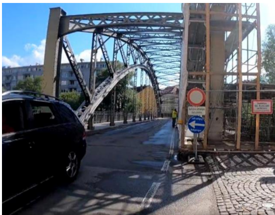
Problematic traffic signs at construction site, with unsafe detour route at EuroVelo 14 in Austria
