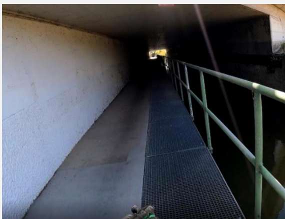
Too narrow bicycle infrastructure at an underpass on the EuroVelo 9, Austria
