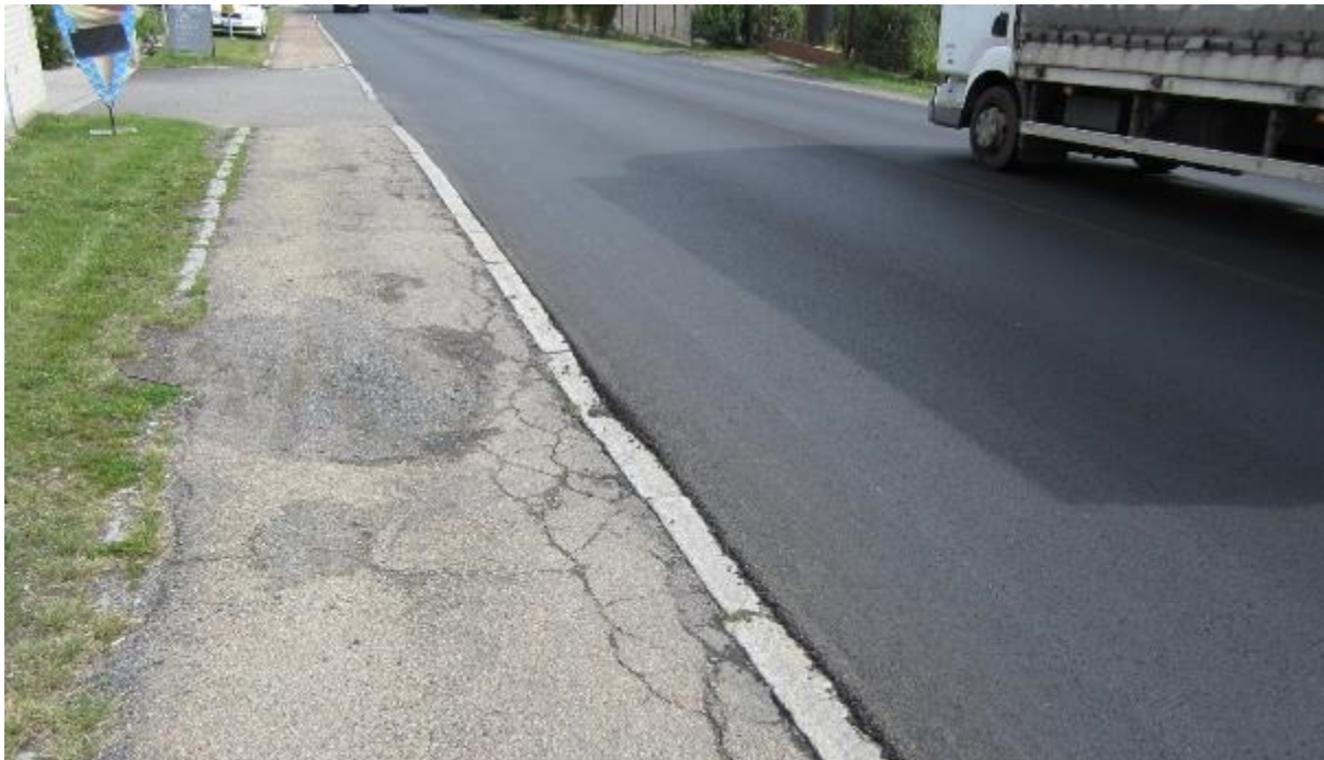
Figure 51 – I/3 through road in Olbramovice – detail of a sidewalk condition – bad surface, levelled with road surface
