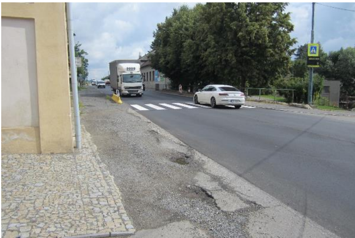
Figure 52 – I/3 through road in Olbramovice – another example of sidewalks condition on a road of international importance
