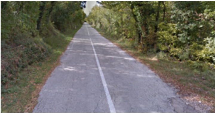
Potholes and damage due to tree roots at EuroVelo 8 in Croatia [12]
