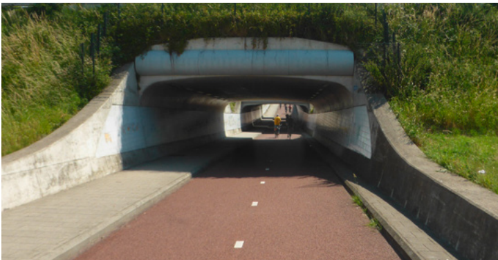
Eisenhower tunnel on the F325 cycle highway, the Netherlands. Straight approach, good visibility and smooth curves at the tunnel entrance, sunlight windows further in the picture [5]
