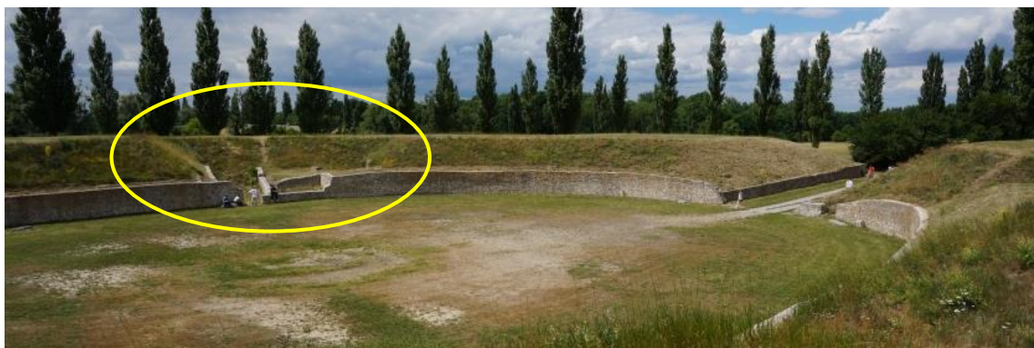
Typical erosion due to action of visitors.
