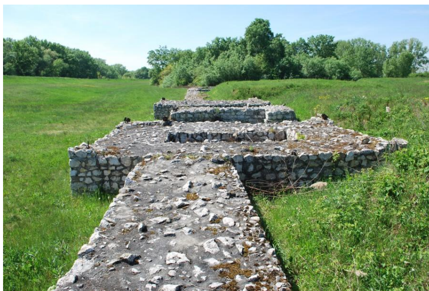
Conserved of historic masonry with hard mortar and compact crown structure (Iža, Slovakia)
