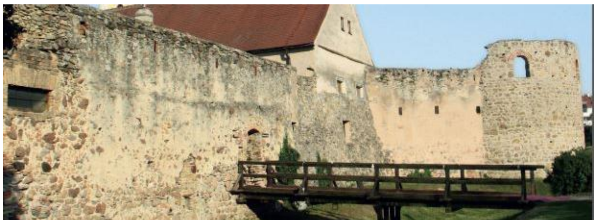
Surface degradation and biofilm on Roman masonry. Melted snow or rain damages masonry with unmaintained top covers which must be kept sufficiently tight. Running water further stains walls and supports growth of bacteria or algae. (Autern, Austria)
