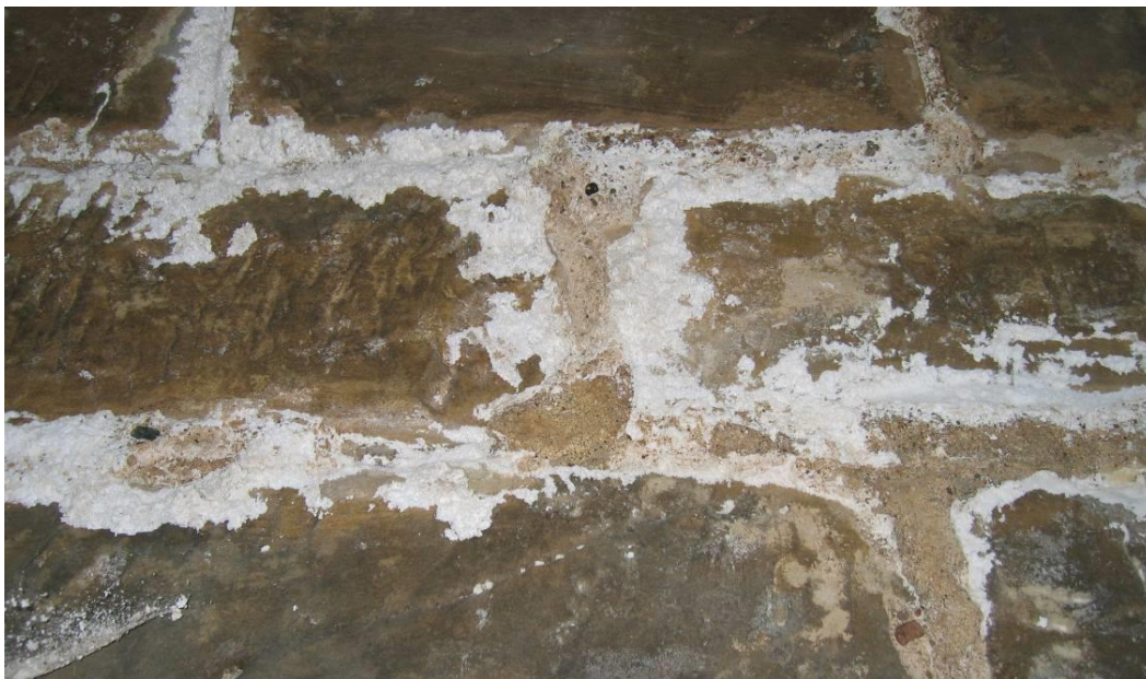
Salt efflorescence appears typically after drying of previously wetted walls.
