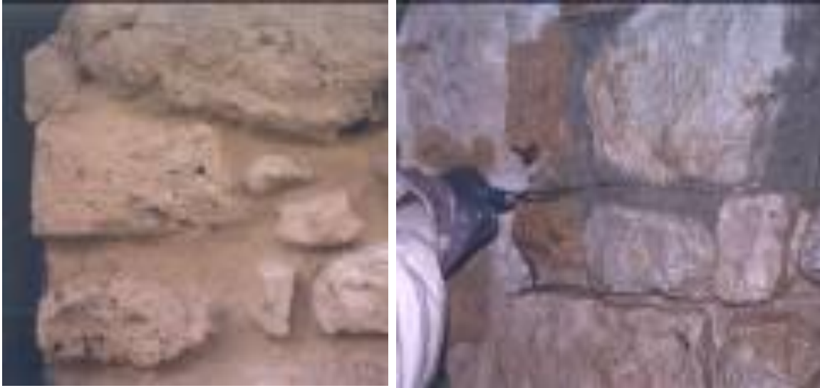
Masonries suffer in mortar joints which need repair of re-pointing.
