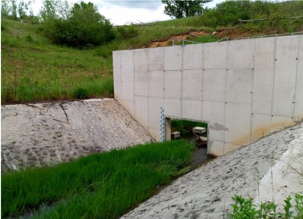
Figure 9. & 10. Road No. 2 crossing of the Hévíz-stream with an inappropriately sized culvert
