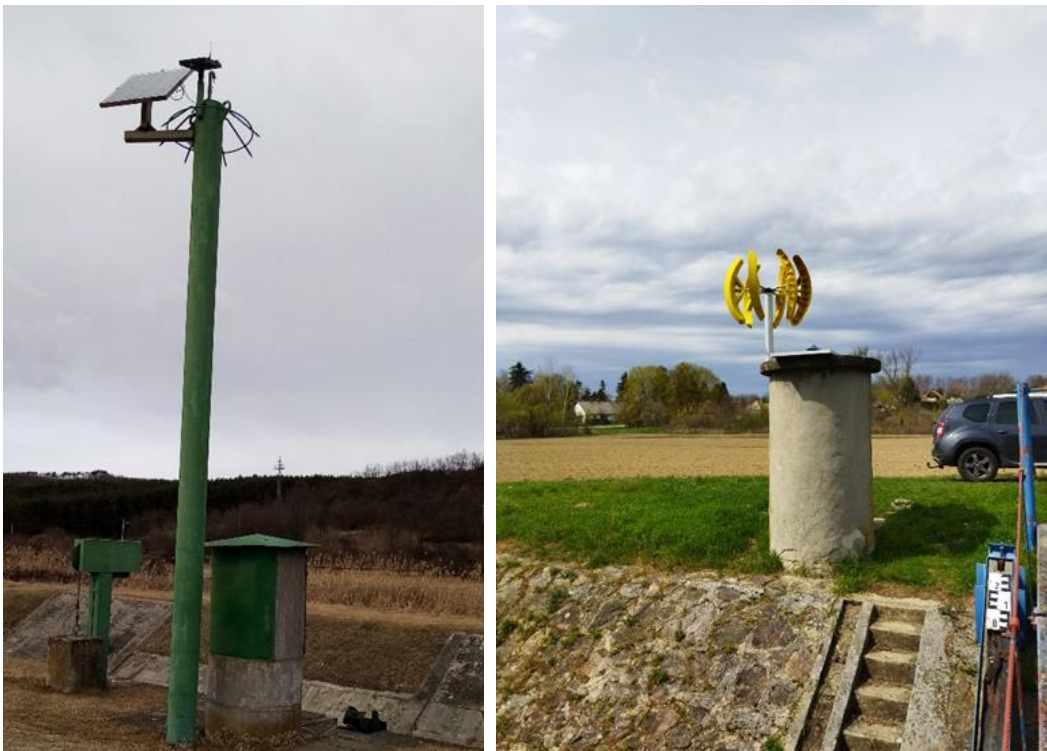
Figure 12: Solar panels and wind turbine installed in Hungarian stations to provide electricity supply for sensors and autosamplers (left: Nemti, Zagyva, right: Törökkoppány, Koppány).
