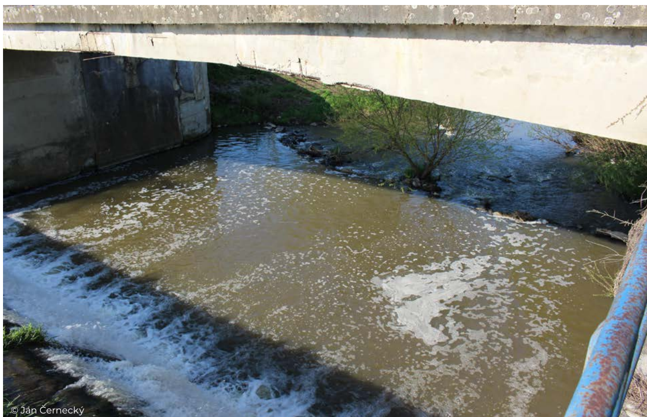
Figure 56 Water impact beam - migration barrier near the village of Holiša - Ipeľ River.
