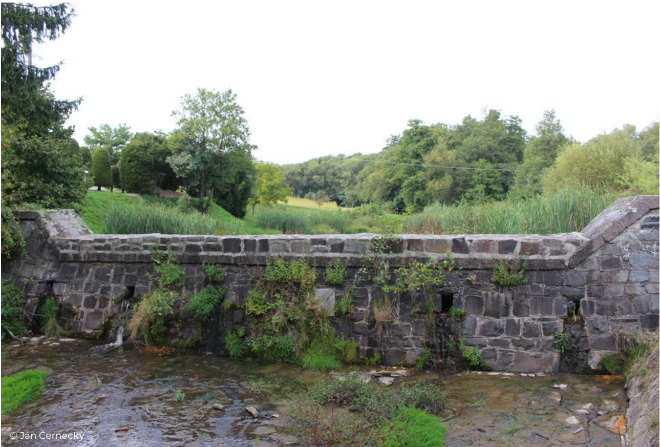
Figure 47 Transverse barrier on the Detsviansky potok brook in the old part of Detva.
