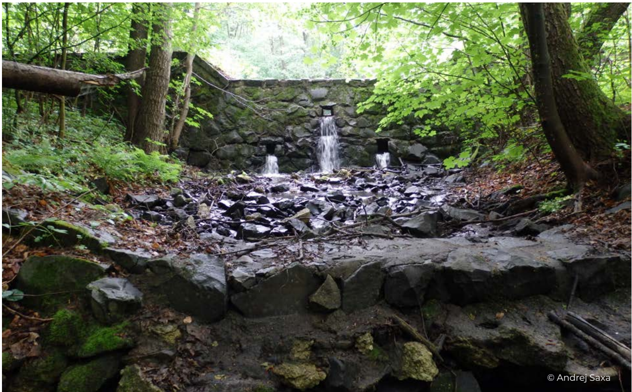
Figure 68 Flood protection dike above the village of Dobroč.
