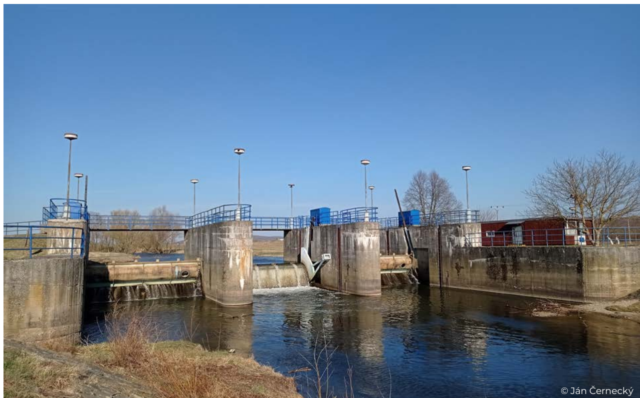
Figure 58 The iron-concrete dam on the Ipel' River is another large migration barrier for aquatic animals, where a suitable solution for aquatic animal migration is completely lacking or insufficient.
