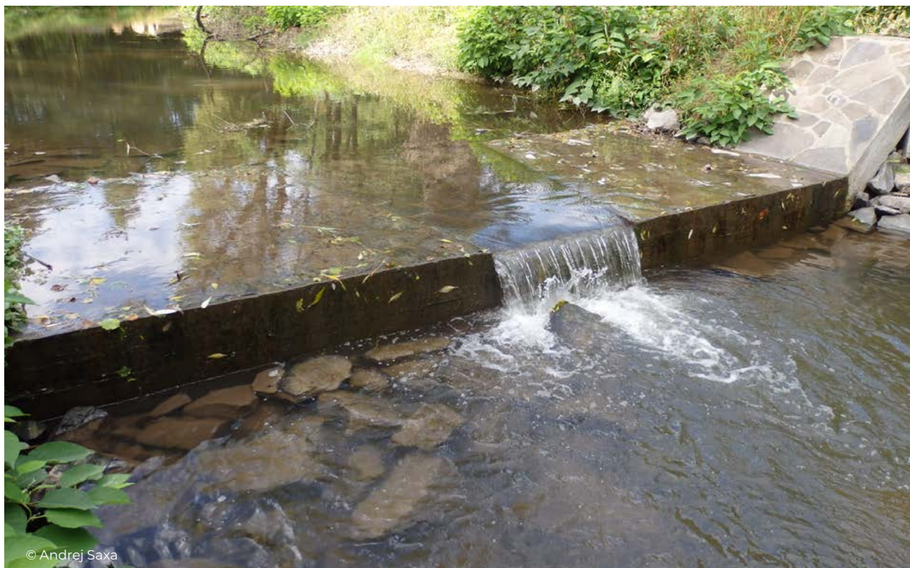
Figure 63 The relatively new, slightly impassable barrier on the Krivánský potok brook above the Mýtina reservoir is problematic for fish and aquatic animals, especially during low water levels.
