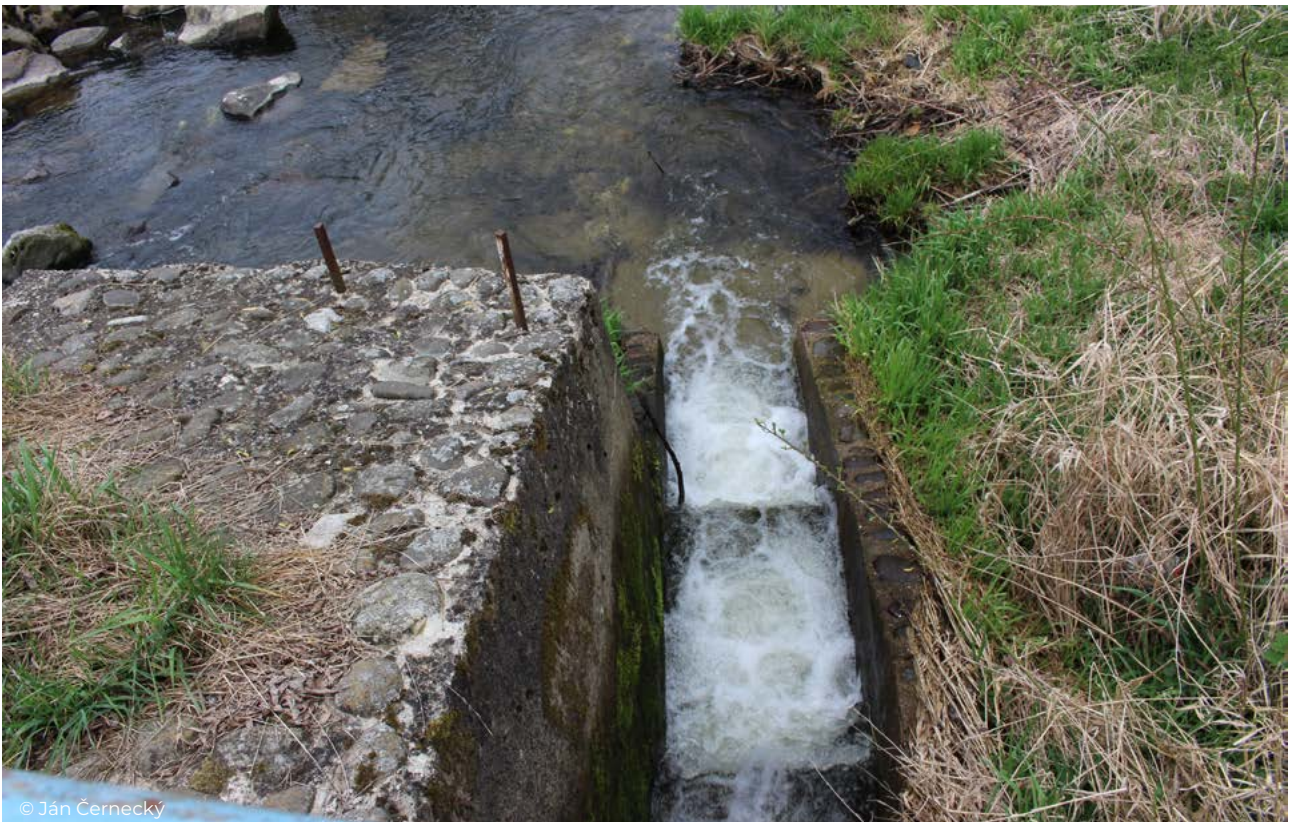
Figure 54 Outlet of the fish passage - Slatina River, Korytárky, flap gate for Korytárky hydroelectric power station.
