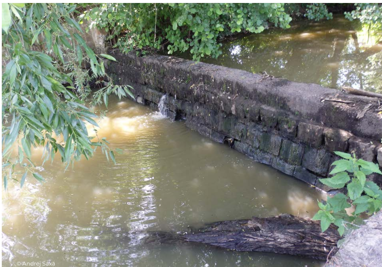
Figure 72 Barrier on the Tuhársky potok brook above the town of Lučenec in the locality of the Parný mlyn.
