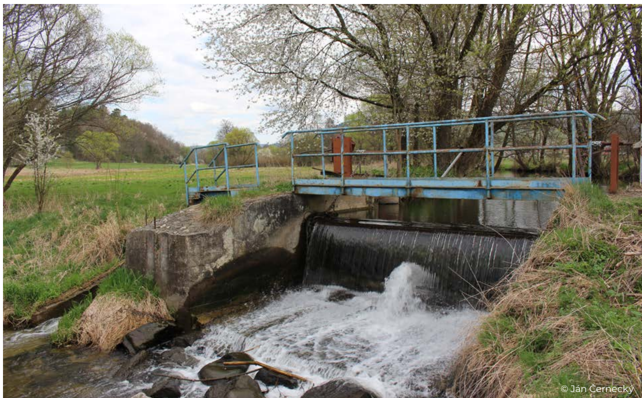
Figure 52 Migration barrier on the Slatina River in the village of Korytárky - it is a flap dam for the Korytárky hydroelectric power station.
