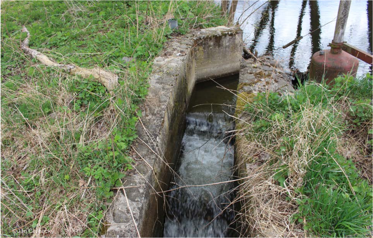
Figure 53 Beginning of the fish passage - Slatina River, Korytárky, flap dam for Korytárky hydroelectric power station.
