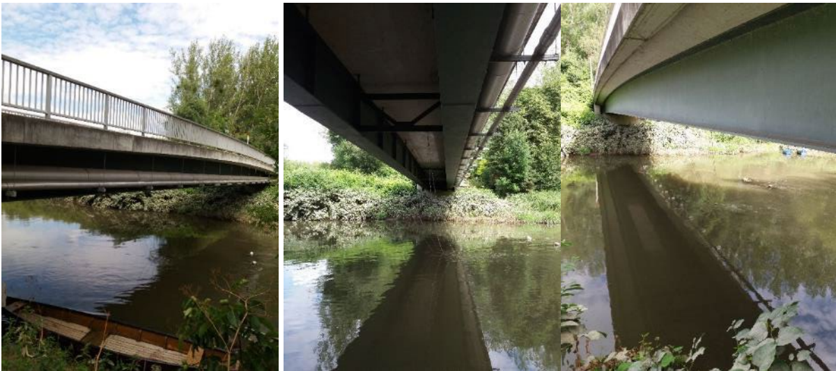
Annex 4: Photos of the installed sedimentation box under the Zaineth Bridge on the Schwechat River
