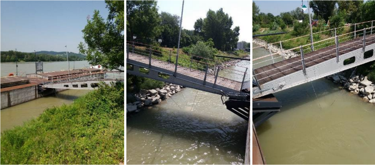
Annex 2: Photos of the installed sedimentation box in Korneuburg
