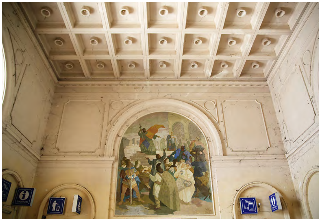
Fig. 191 / Giurgiu railway station in a neglected state (Author: C. Vărzaru)
