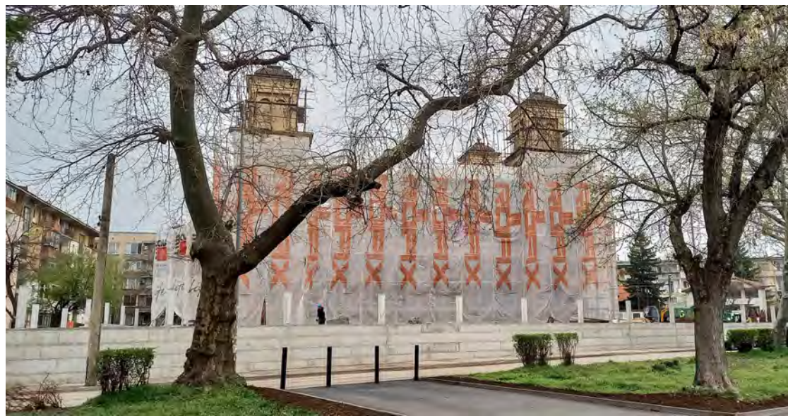
Fig. 295 / The refurbishment of Vidin synagogue on the Danube riverfront historic promenade (Author: G. Georgiev)
